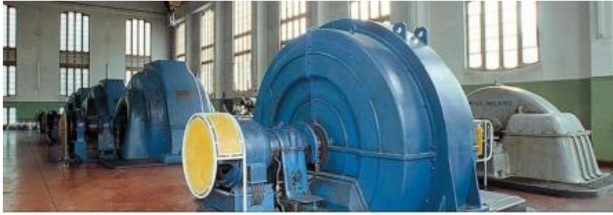
Figure 48. Image hydroelectric power plant operated by BIM.
